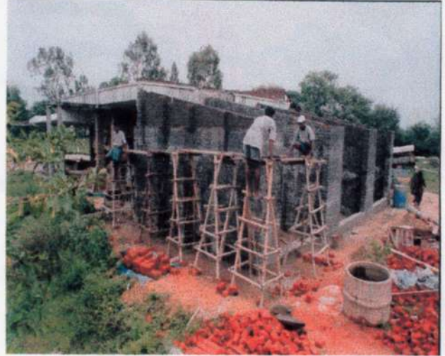
Masons completing the walls for new storerooms on the back of the godown
